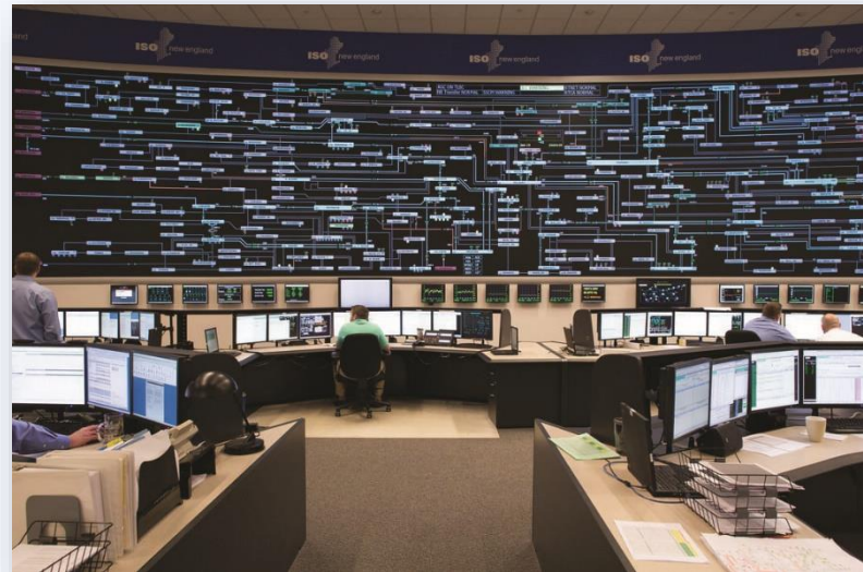
(ISO-NE Control Room)
